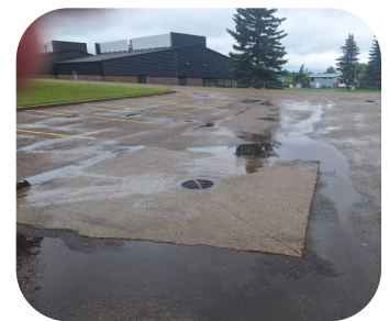
Catch basin (drain) with concrete perimeter
